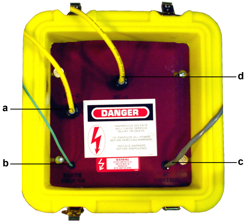
Figure 3. High Voltage Module
